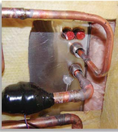
Figure 4. Refrigeration Line Sleeves
